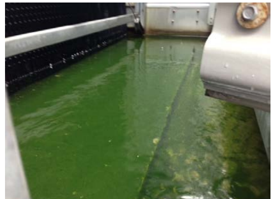
Figure 6 Algae growing in cooling tower water. Photo courtesy of LinkedIn .
