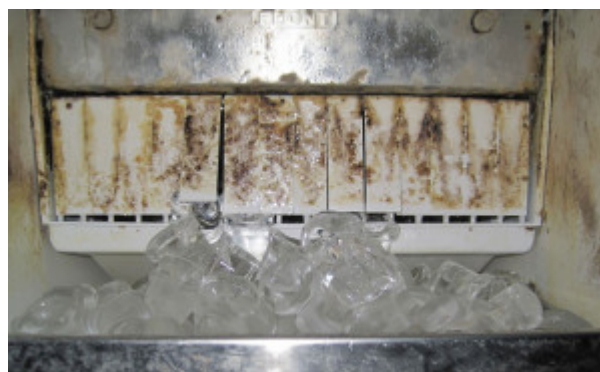
Figure 12 Mould and rust in an ice machine
