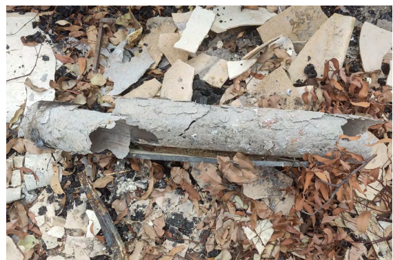
Figure 7 Fire damaged asbestos cement flue.
